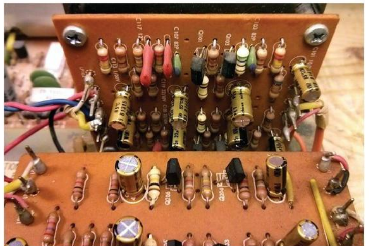
The tone and phono boards showing new Nichicon Fine Gold audio-grade electrolytic capacitors.
